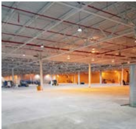
As the project progressed, you could see the previous yellow-tinged lighting side-by-side with the new brighter, whiter energy efficient LED lighting.
