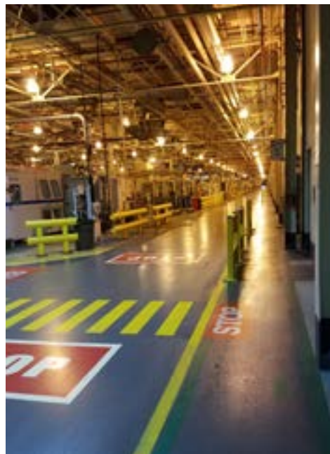
Before the LED retrofit.
